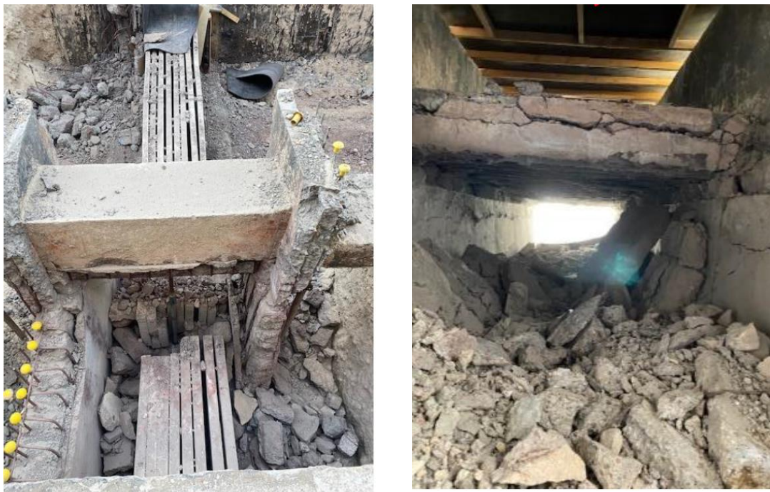
Figure 9. Root cause of Eagle incident. Left: busbar cut off in east tunnel. This was the first event. Right: lower ceiling (of double ceiling) decomposed and collapsed onto the busbars in east tunnel.
