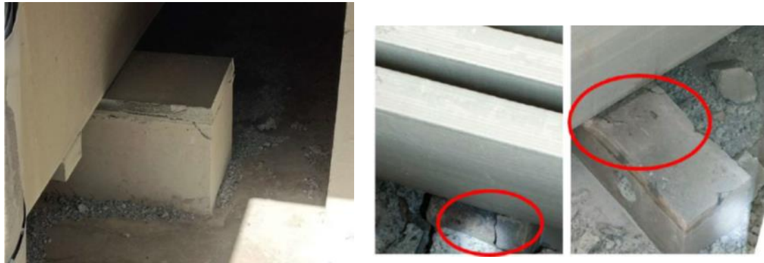
Figure 5. Typical damage to the busbar supports. Left: detachment of epoxy grout; this does not need repair. Right: Cracks that were recommended for repair, even though they do not compromise busbar integrity.
