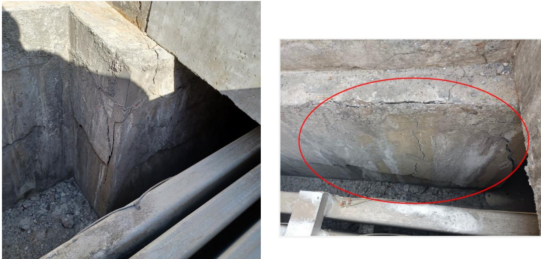
Figure 7. Damaged tunnel walls in Potline 6 south below the gantry road, which had to be rebuilt.
