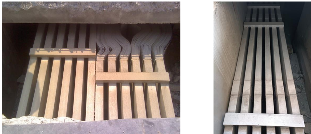
Figure 4. Busbars displaced by attractive electromagnetic forces; left - 2 packs in one tunnel, right – 2 packs in different tunnels. Tie-bars were not damaged.
